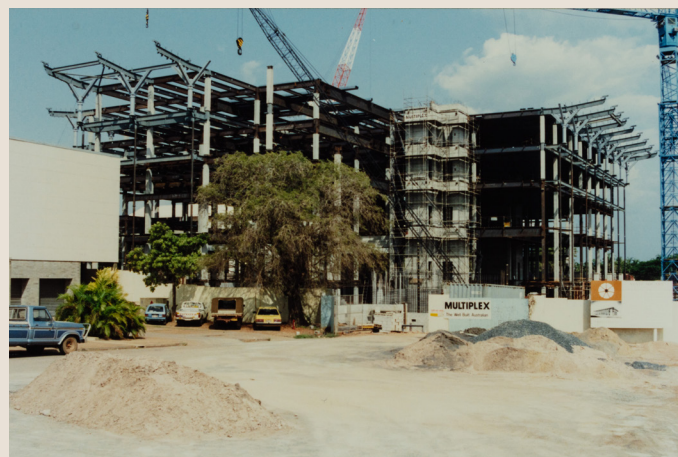
Construction of Parliament House, Darwin. Image courtesy of Library & Archives NT, Libraries 1991-1992 Collection, Image PH0427/0169, https://hdl.handle.net/10070/330466 .
